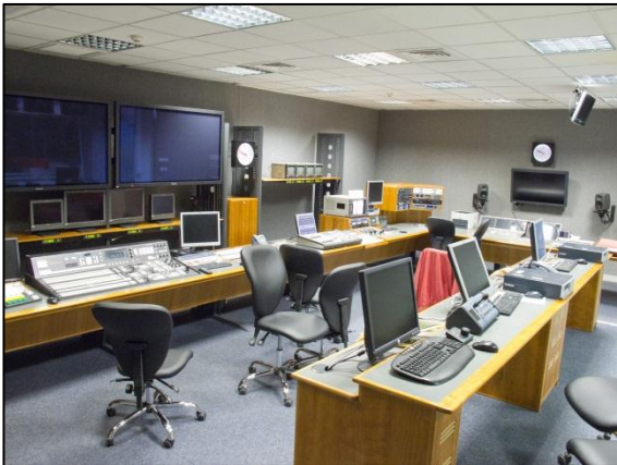
Figure 3 Well equipped Production and Lighting gallery
